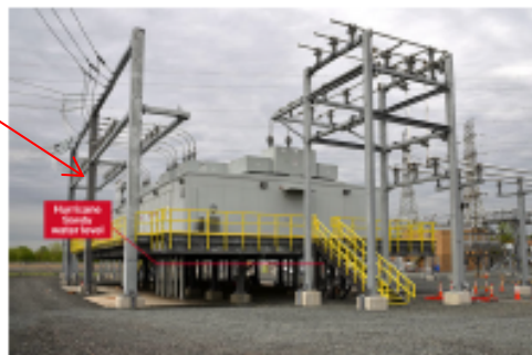
A PSEG Power substation in Sewaren
